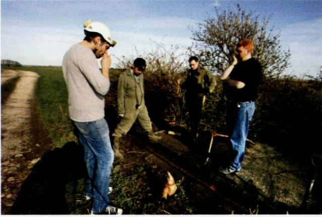
brickwork pillars. They also put three large cracks across the face of the slab.
